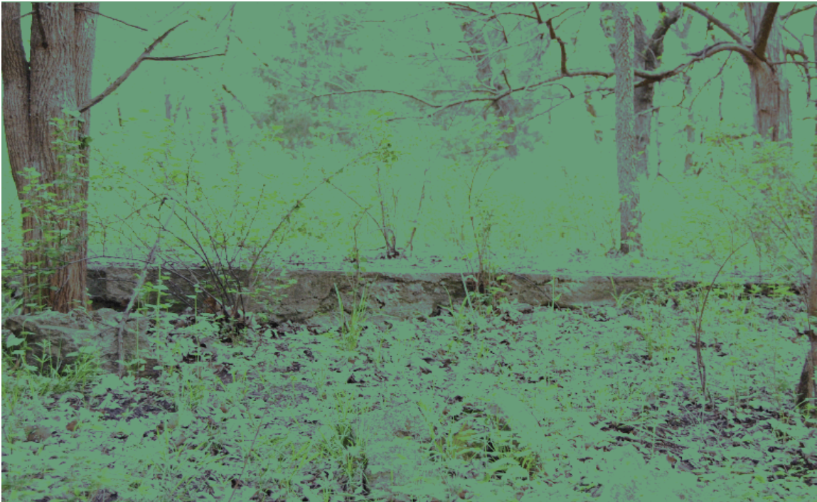
Figure 3: Photograph of the concrete foundation in its current state. Deterioration is visible in the form of cracks that run along the edge of the slab. SOURCE: Photograph courtesy of Jim and Marian Bradley.
