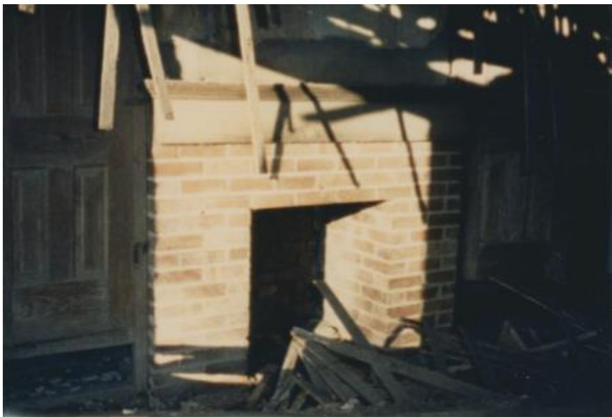
Photograph of the inside of the stone house in 1988. The signs of decay are more prominent from this view of wooden pieces that fell to the floor. Photograph courtesy of Barbara Booth.
