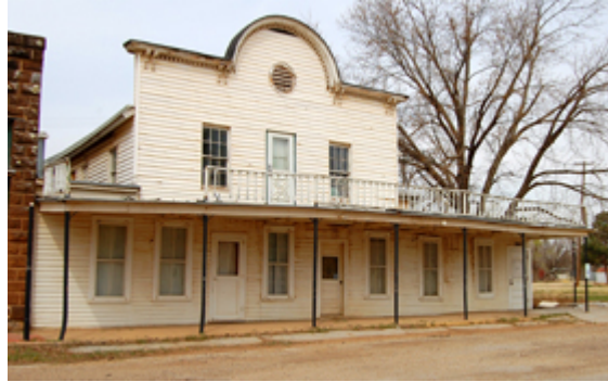
Figure 2: Here is a photograph of the original Brookville Hotel. As you can see it is now vacant and run down. Photograph taken by and accredited to Kathy Weiser. March, 2009
