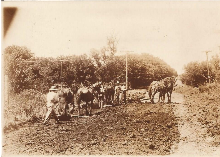
Figure 4. Photograph showing a road being built near Goff, Kansas, c. 1915. Roads like the Great White Way would have been built in a similar way, with the poles in the distance painted with bands of white to serve as a guide for drivers. SOURCE: Personal collection of Roy Bell
