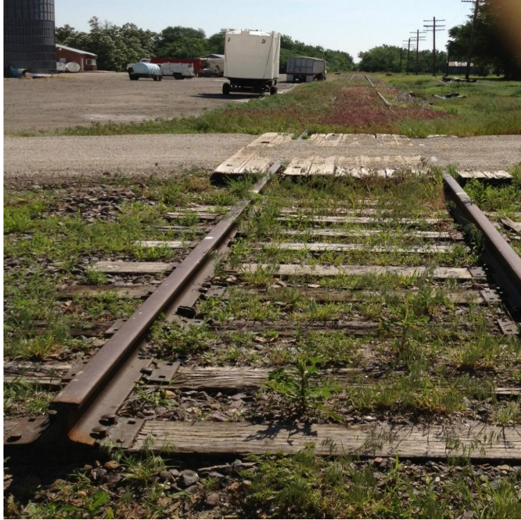
Figure 3: This is a picture of the abandoned Missouri Pacific Railroad tracks in Hope. Once a very important factor in the Hope community, the line now sits unnoticed in the community's backyard. Photo by author, April, 2012.
