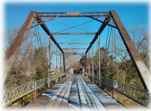
Figure 6. Photograph of the current condition of the Bodarc bridge, c. 2013 SOURCE: Personal collection of Evan Voth Notice the durability of the iron 128 years later.
